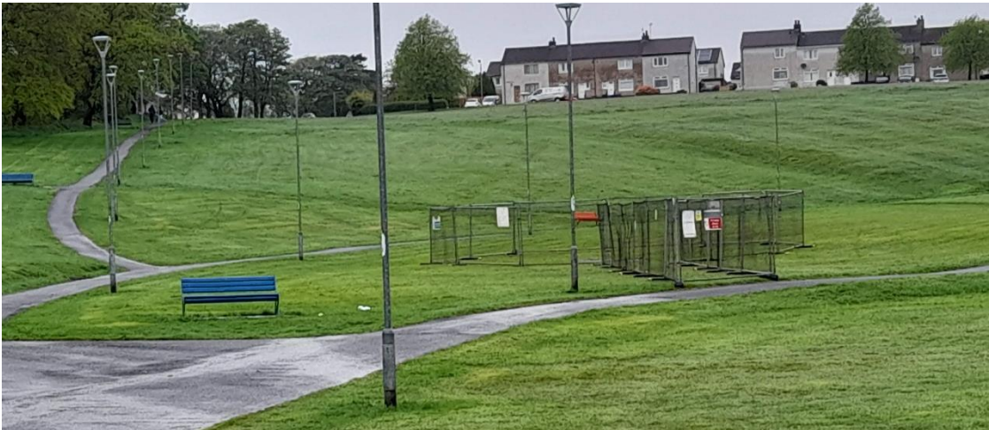
Getting ready to start installing stones in a circle at Kilbirnie Public Park
